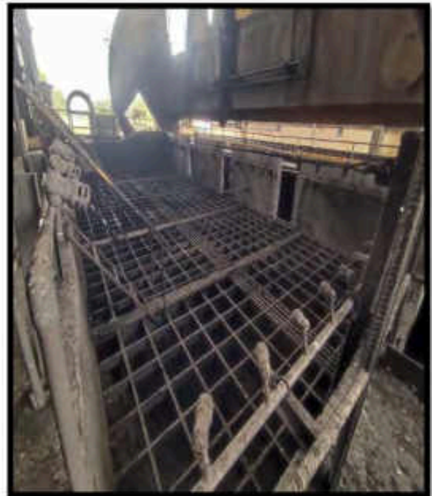
Water Sprinklers in Wagon Tippler
