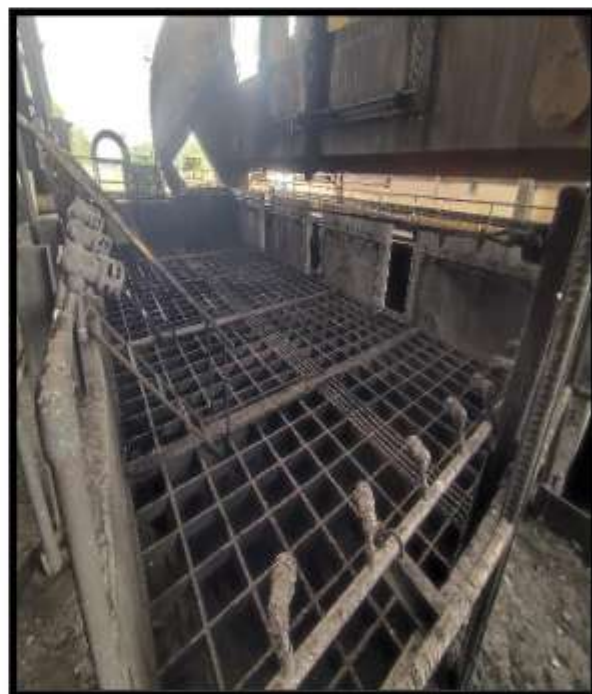
Water Sprinklers in Wagon Tippler
