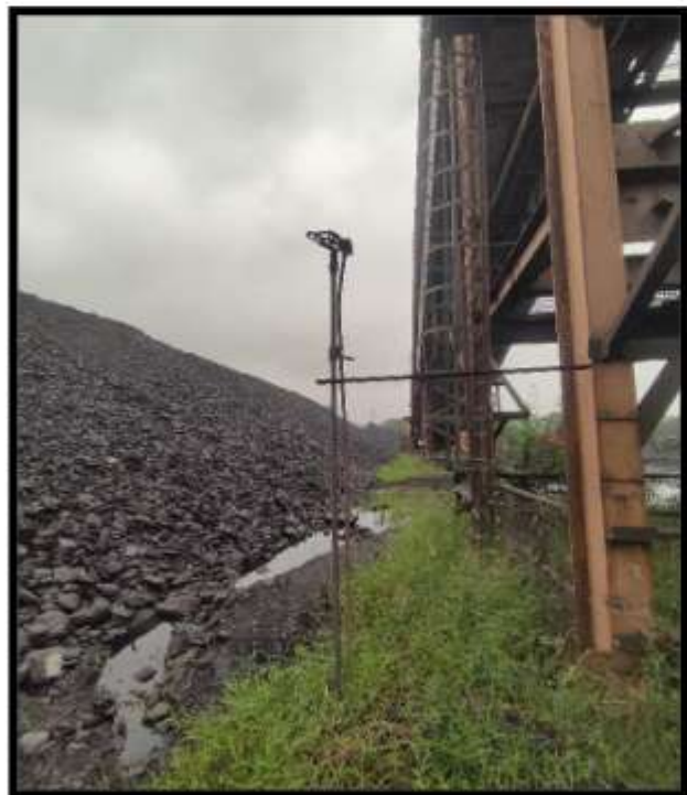
Water Sprinklers in Coal Stock Area
